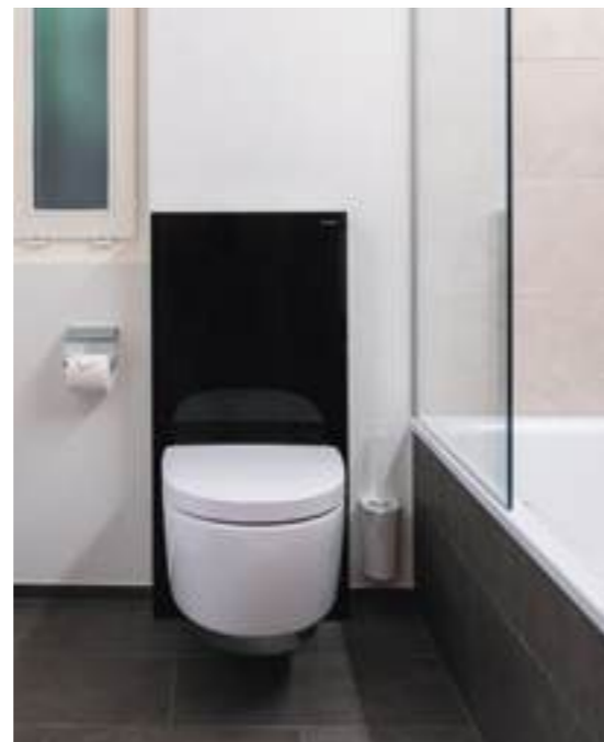
AFTER Installation situation with Geberit Monolith
