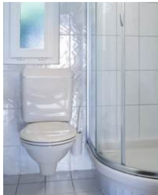
BEFORE Installation situation with exposed cistern
