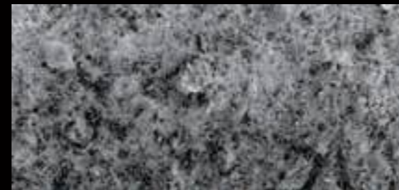
Grout in the tiled area rough, porous
